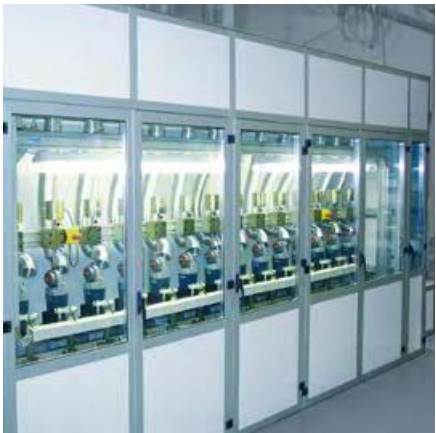
Protective cabinet and noise protection
