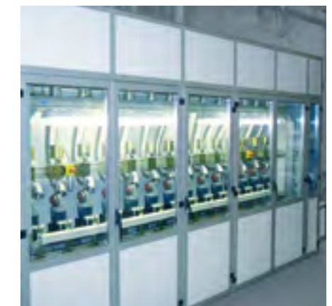
Protective cabinet and noise protection
