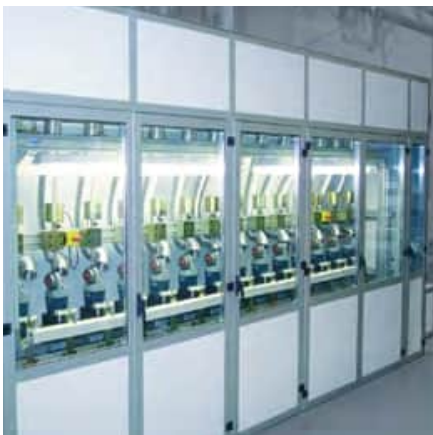
Protective cabinet and noise protection
