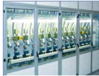
Protective cabinet and noise protection
